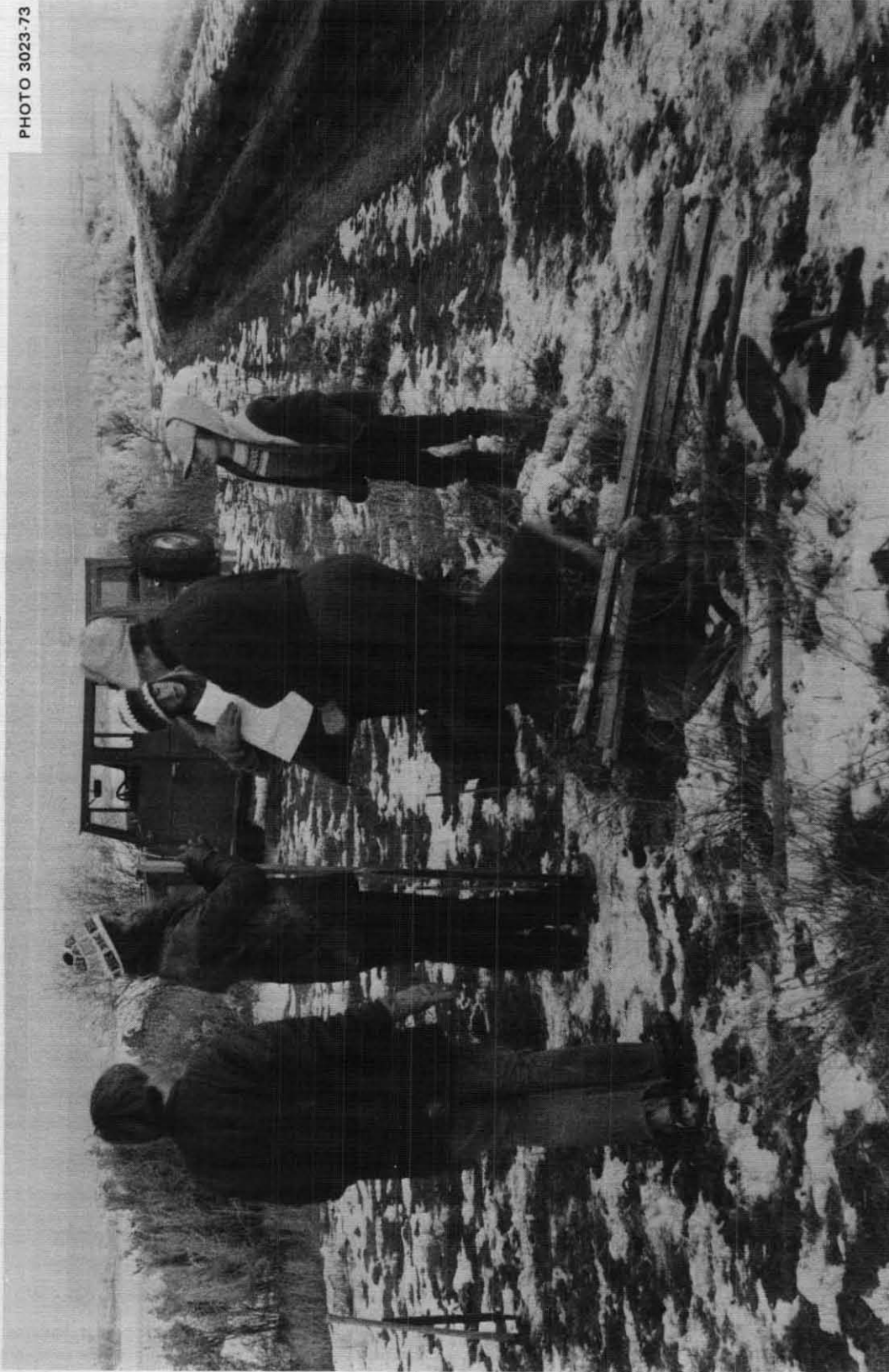
Fig. 2.2. Starting to stake out the shelter trench near Montrose, Colorado, at 7:17 AM. The six doors, some tools, water, etc., were carried in a station wagon. The ground was frozen only about an inch deep.
